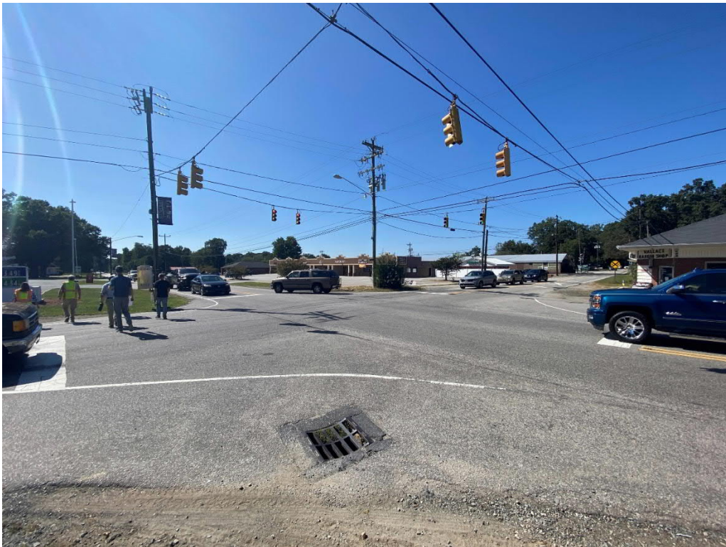
Stormwater drainage inlet located at the intersection of NC 75 and Potter Road.
