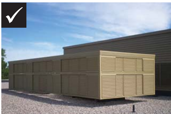
Screened roof-top equipment
