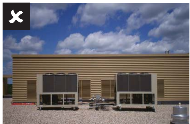
Unshielded roof-top equipment
