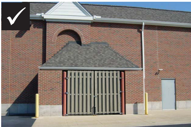
Screened ground-level equipment
