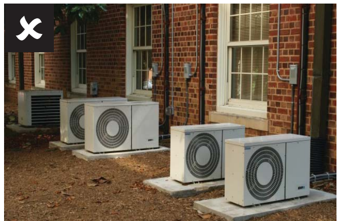
Unshielded ground-level equipment
