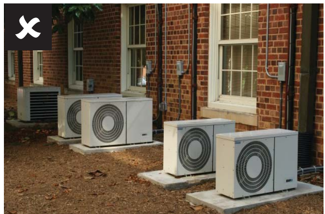
Unshielded ground-level equipment
