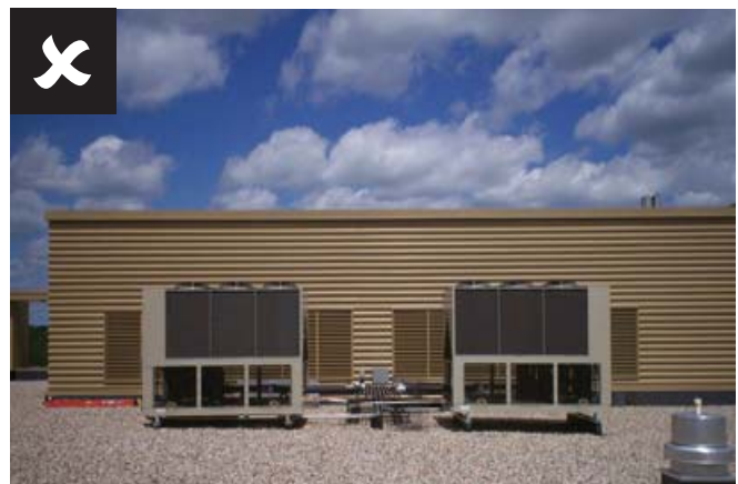
Unshielded roof-top equipment
