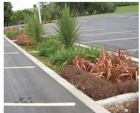
Recessed curb with sheet flow drainage to landscaped area
