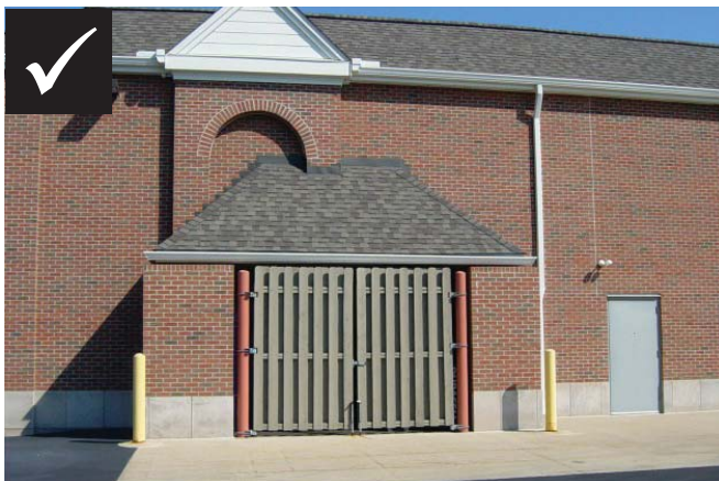
Screened ground-level equipment
